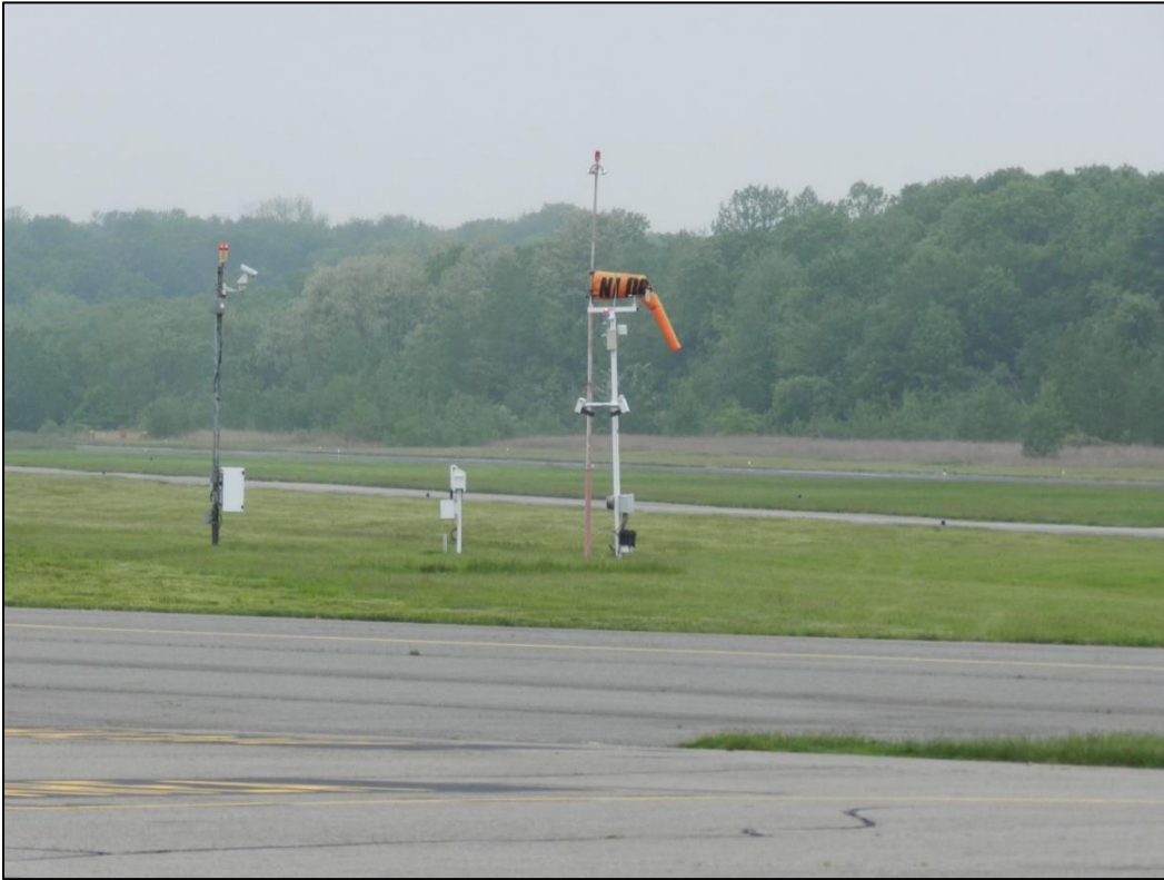
Figure 4-14. Existing Wind Sock and AWOS Within the Primary Surface with Obstruction Lighting
