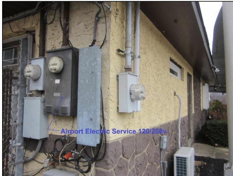
Figure 3-33. Airport Electrical Service Entrance
